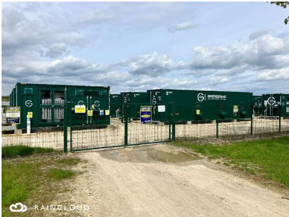
Plate 12-21 Typical Corner Pads and racking on BESS units
